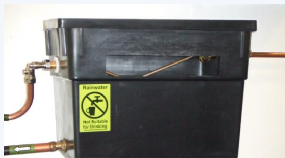
Figure 3: examples of labels for storage cisterns and point of use appliances e.g. washing machines, WCs, outside taps etc.
